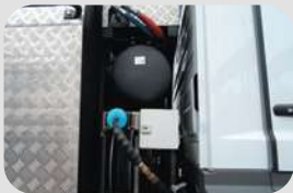
Hot-water cleaning systems
